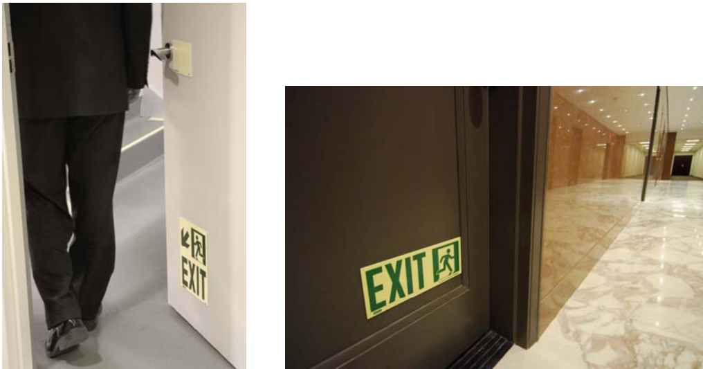
Exhibit 3: Stairwell entry doors showing low placement of the photoluminescent emergency exit sign.
