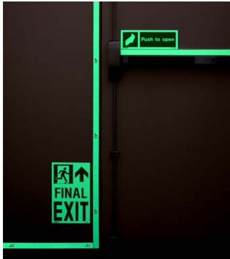
Exhibit 10 Final Exit door showing mandatory sign, perimeter marking, pushbar marking, and optional “Push to open” sign.
