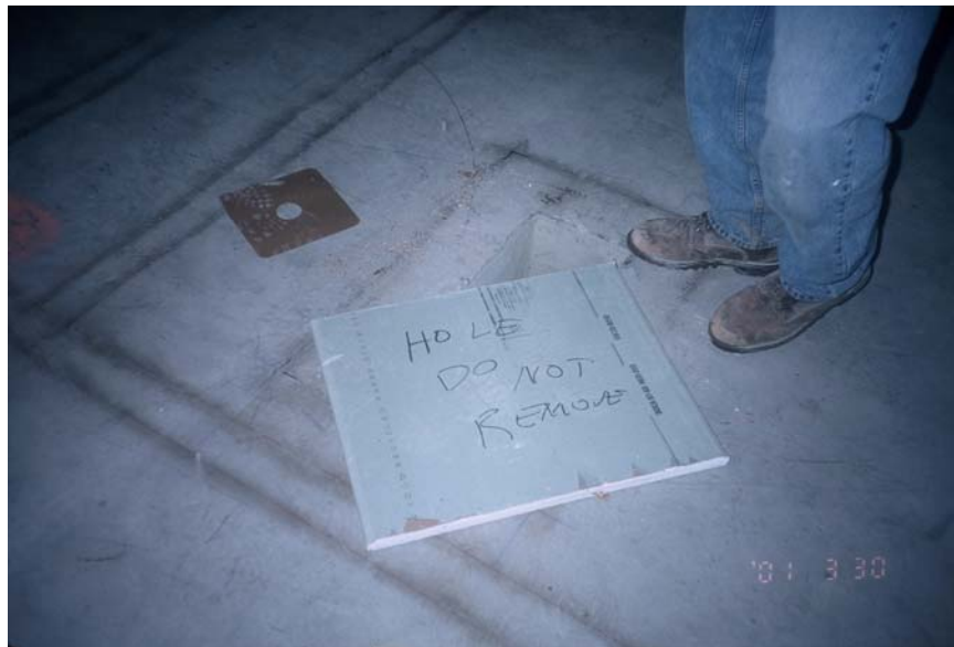
Exhibit 5: Sheetrock Floor Hole Cover – Twice the Intended Load?
