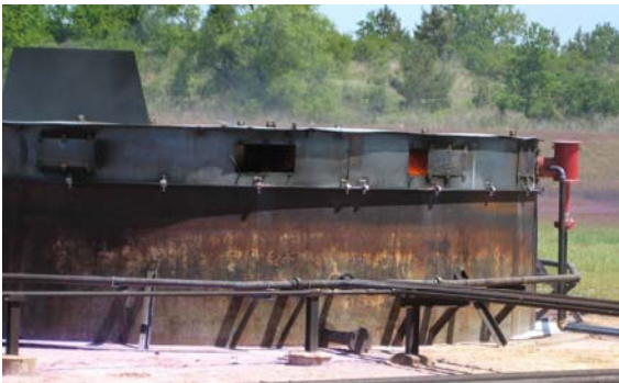
Exhibit 15 Residual appurtenance fire shows through RH vent after foam puts out most of the fire. Note: where there was smoke there was fire.
