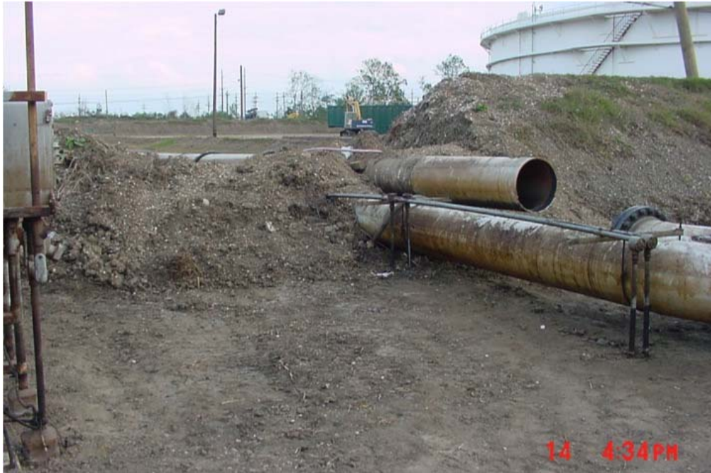
Exhibit 7. The oil escaped through this failed section of containment berm.
