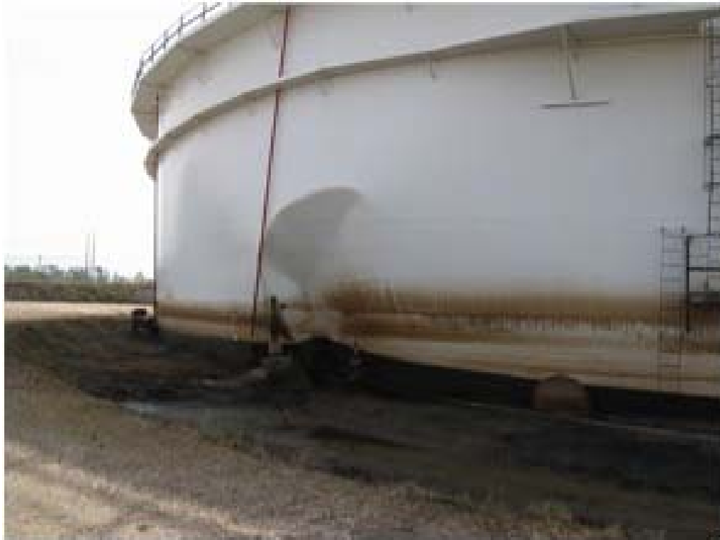
Exhibit 6. This is the “crumple zone” leak.
