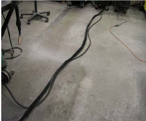
Figure 4. Welding cables stretched across the floor, causing a tripping hazard.
