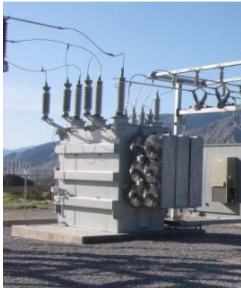
Figure 3: Typical Substation XFMR
