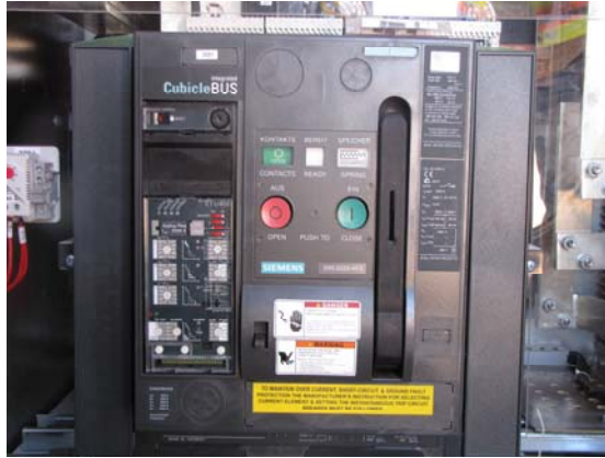
Figure 4: Low Voltage Power Circuit Breaker.
