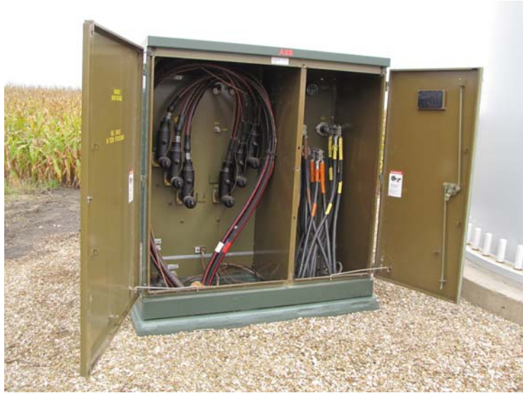
Figure 2: Typical Padmounted XFMR
