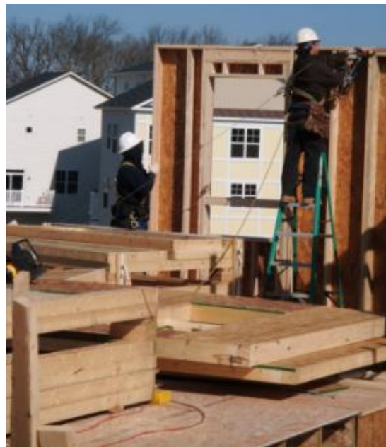
Exhibit 11. Framers installing second floor walls using self-retracting lines and anchor points installed on floor.
