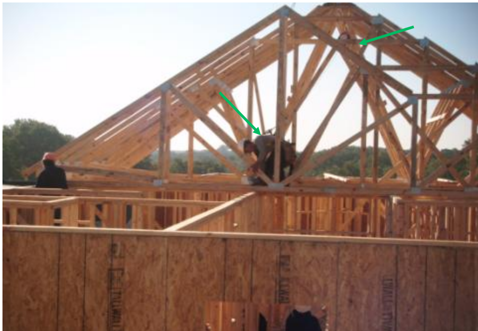
Exhibit 16. Worker using self retracting line and anchor point installed in trusses to set trusses
