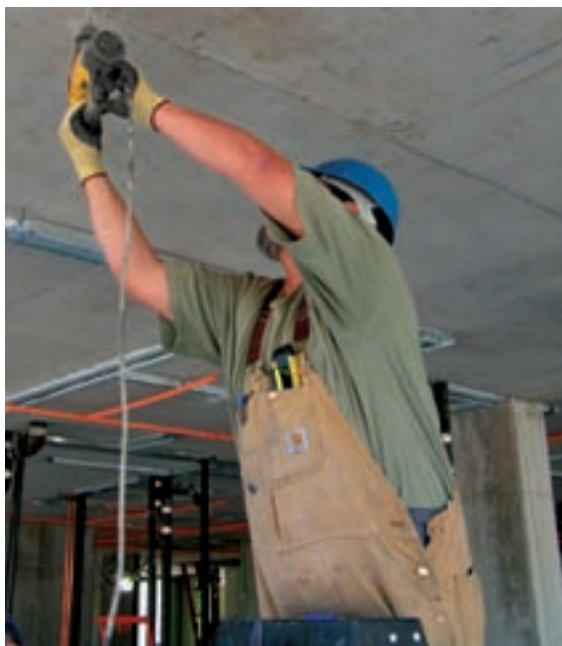
Photo 1 (top): A contorted neck posture is common during the usual method for overhead drilling. This construction worker is wearing eye and hearing protection but not respiratory protection for possible dust/silica exposure.
