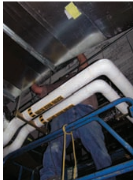
Photo 11 (left): An inverted drill press column with a 4 ft extension threaded between conduits. The device is being operated from the ground.
