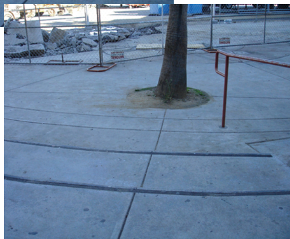
Photo 2: This half-round stair has an unusually long tread. The step edges could be made more conspicuous with hazard yellow striping and an intermediate handrail. Also note the deceptive visual cues created by nearby expansion joints, and the adjoining ramp handrail (to the right) which is excessively long.
