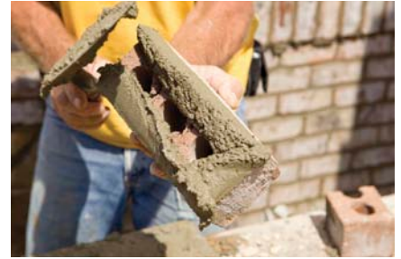
Buttering—applying and smoothing mortar using a trowel—is one of seven risk factors for back and shoulder injuries for all masons.
