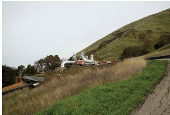
Photo 5: WSIP Alameda Siphons Ventilation.
