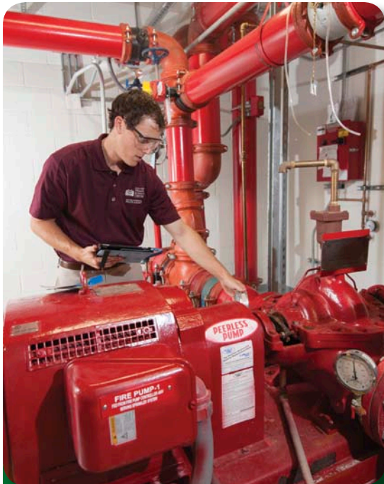
Nathan Jennings, TAMHSC assistant fire marshal, inspects a fire pump using an iPad.
