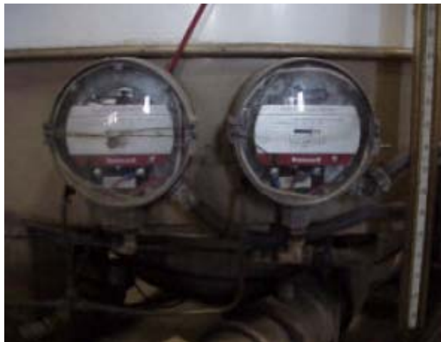
Exhibit 5. High/low gas pressure switches verify gas pressures are in the proper range.
