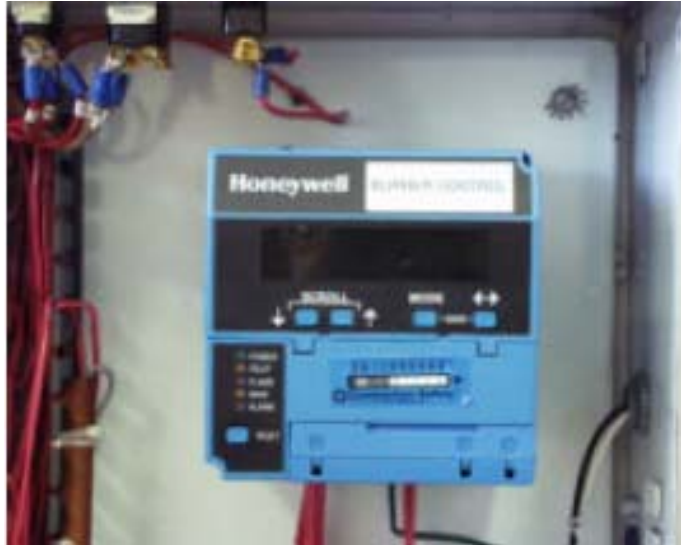
Exhibit 6. The burner management system (BMS) is the “brain” that monitors/directs safe firing and operations.
