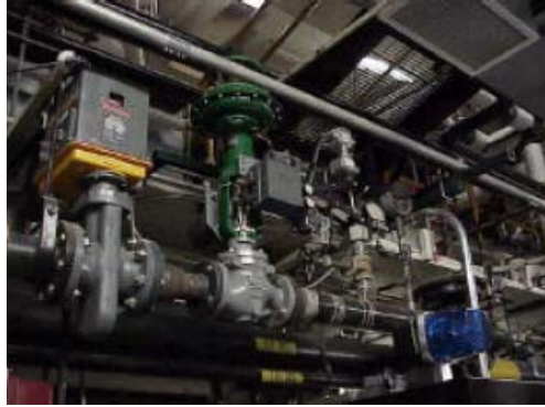
Exhibit 3. This is a typical gas train with safety interlock components.
