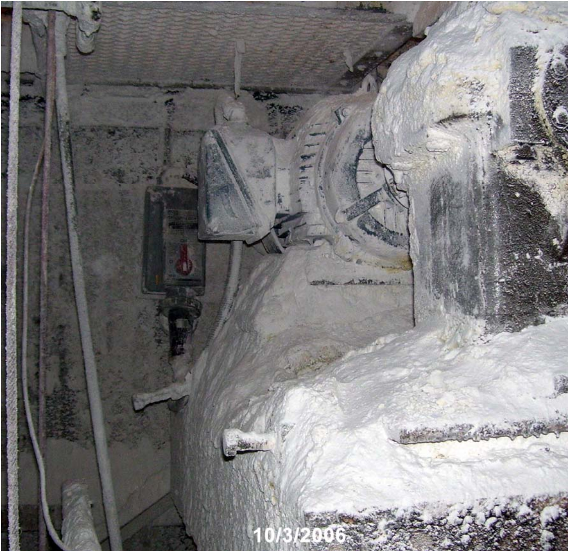
Exhibit #4. Housekeeping conditions such as this may lead to a major loss incident. Photo courtesy US Chemical Safety and Hazard Investigation Board.
