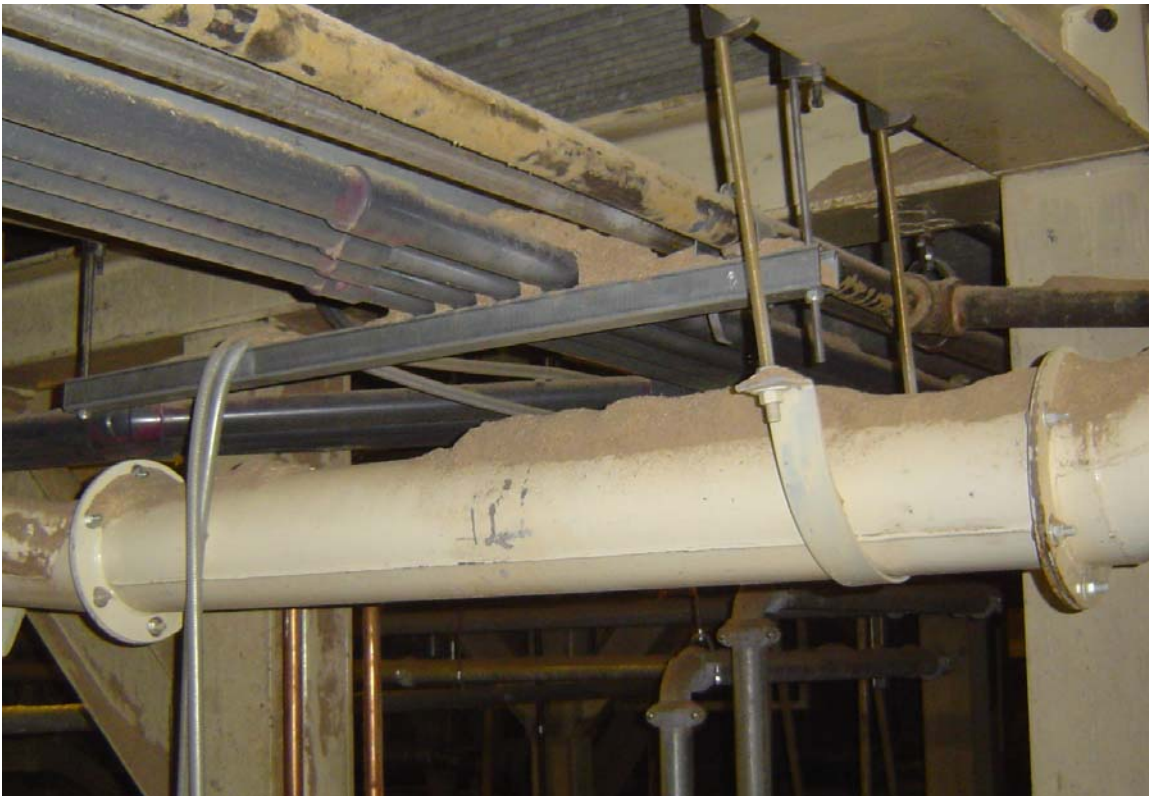
Exhibit #3. Ducts, conduits, and building members should be maintained free of dust accumulations.
