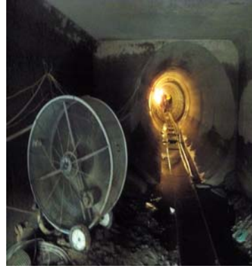
Exhibit 8. 4-foot ventilation fan.
