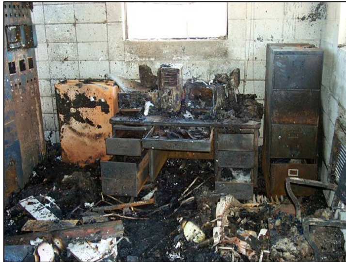
Figure 4. Switchgear Room Post-Arc Flash and Fire.
