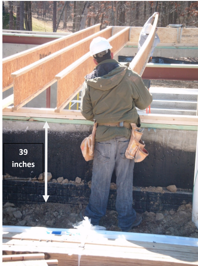
Exhibit 7. Framers installing floor joists from backfilled ground 39 inches from top of basement wall to ground and ladders.
