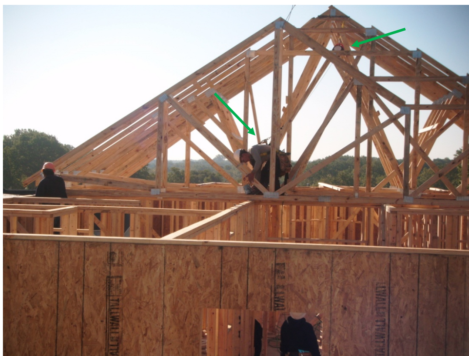
Exhibit 16. Worker using self-retracting line and anchor point installed in trusses to set trusses.
