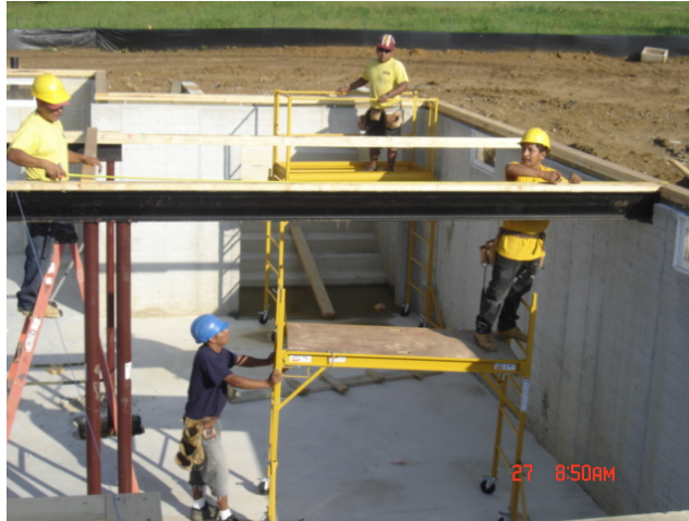
Exhibit 5. Workers setting sill plate on basement walls from ladders and mobile scaffold
