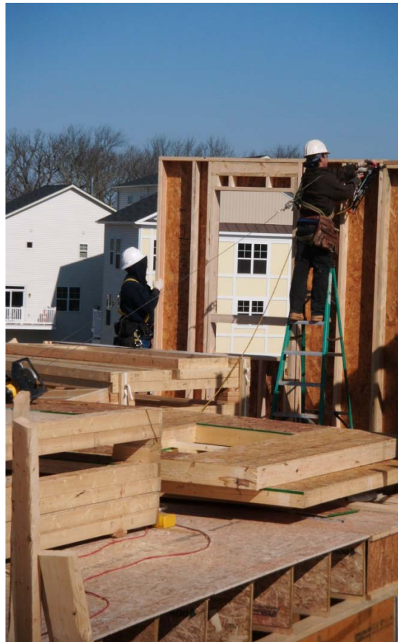
Exhibit 11. Framers installing second floor walls using self retracting lines and anchor points installed on floor.
