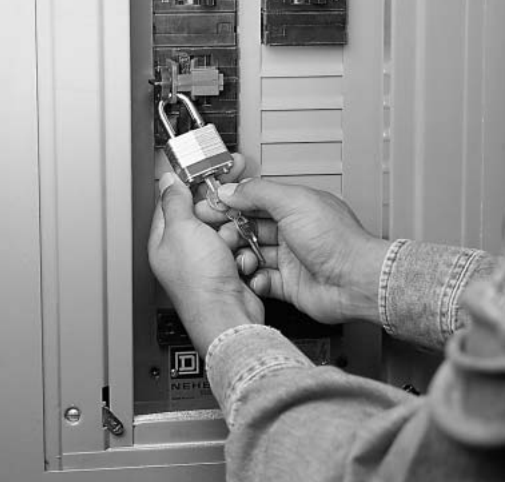
Lockout/tagout at a circuit breaker.
