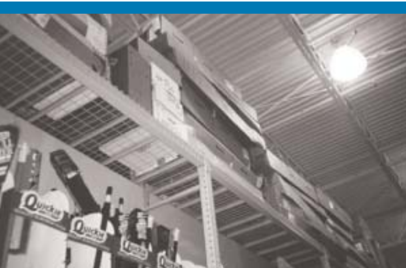
Photo #4 (above) shows cartons on the top shelf that have collapsed.
