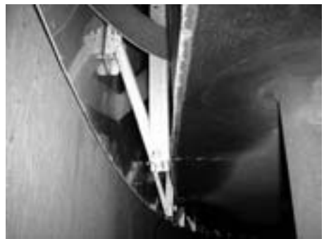
Photo 1 (top): The aftermath of the fire in tank T-1001.
