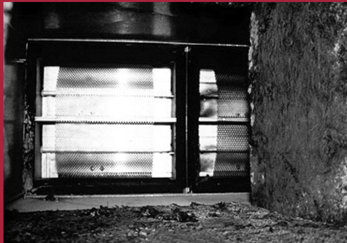
A small amount of visible mold or transient odors may signal greater infestation hidden in various areas, including air ducts (left), air diffusers in the ceiling (below, left), and behind and/or between wall components, such as wallpaper (below, right).
