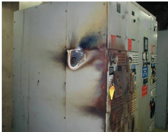
Arcing faults in electrical equipment can create hazard exposures. This photograph illustrates burn through in the left side cover and venting of hot gases around door edges and ventilation ports on the front of the switchgear. (Photo courtesy of DuPont)
