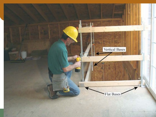
Photo 9 shows the flat and vertical bases being used to install temporary guarding around a large floor opening.
