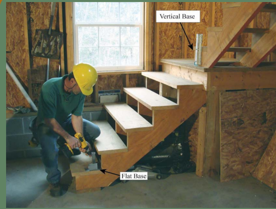
Photos 7 and 8 show the flat and vertical bases being used to install temporary handrails for stair construction. When either of these bases is installed on site, proper fasteners must be used and must be correctly and securely inserted.
