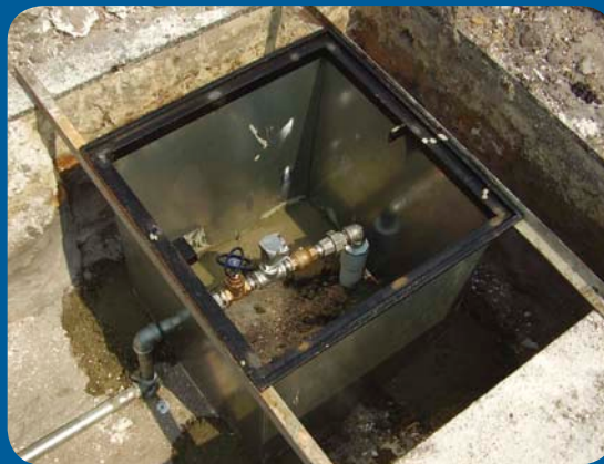
Photo 6: Trenching at a site for constructing vault boxes for remediation systems can pose a safety and health hazard to pedestrians, and pose a threat to unmarked buried utilities.
