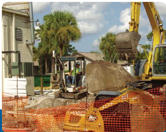
Photo 3: Environmental remediation often involves excavation. During this project, several pieces of heavy earthmoving equipment were operating at once, posing an increased risk from a safety and health perspective.
