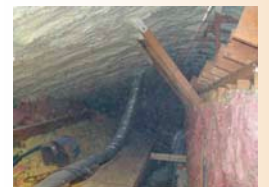
From top: Metal grating (Photo 1) controls expansion of foam, while air movers (Photos 2 and 3) can be used to exchange air in the spray zone.
