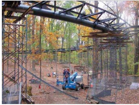
Canopy Steel Bridge (575 ft long and 11 to 18 ft wide) was under construction when it collapsed (Photos 11 and 12).
