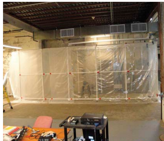
NIOSH has constructed a prototype spray booth (Photo 4, front view).
