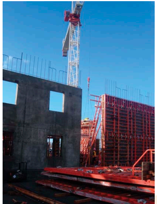
Use of a prefabricated formwork system (Photo 2) can lead to improve safety on construction sites.
