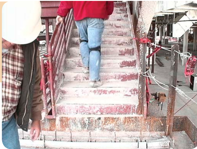
Photo 1: Preinstalling handrails where possible eliminates issues with temporary protection and improves overall safety.
