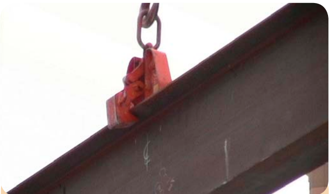
Photo 2: Alternatives to walking the steel can improve efficiency while greatly reducing risk to workers.
