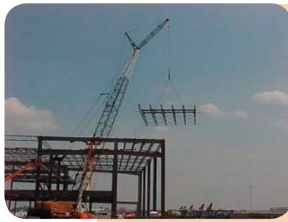
Photo 3 (far left): Use of aerial lifts eliminates some walking the steel needs while greatly increasing productivity and safety.
