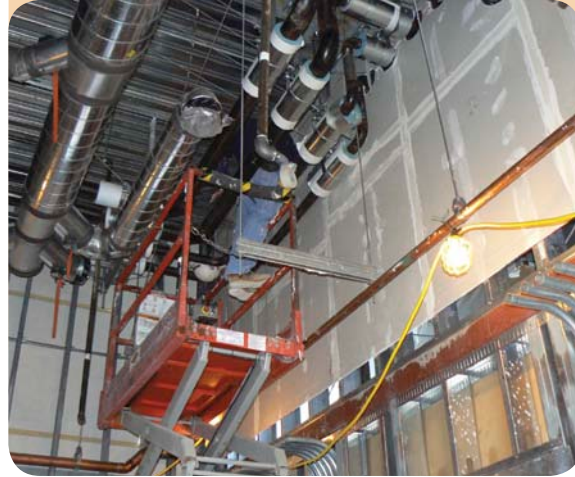
Photo 5: Use of 3-D modeling by a general contractor in work sequencing improves job coordination, subcontractor efficiency and overall job safety.
