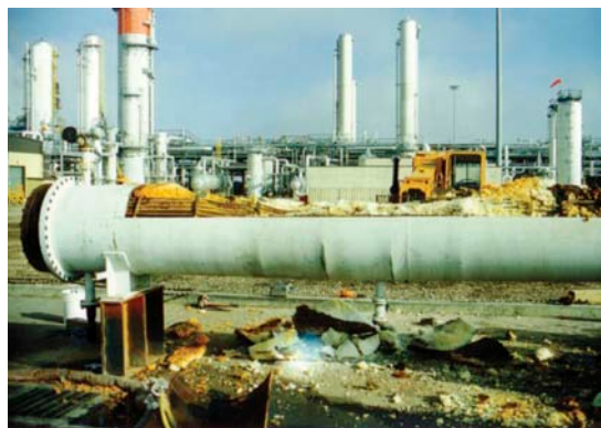
Photo 6: Deformed condenser shell.
