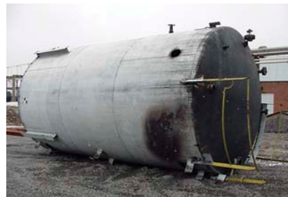
Photo 1 (above): Atmospheric storage tank following the fire.
