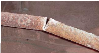
Photo 11 (top): Plant air piping in utilities building.
