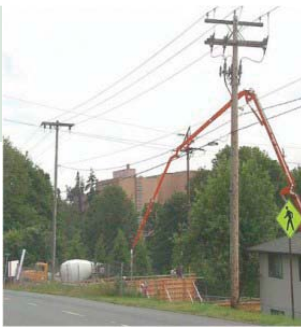
Photo 4 shows a dangerous electrical hazard.
