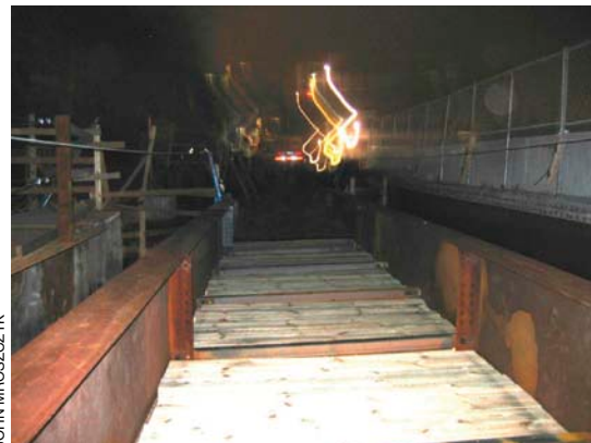
Photo 6 is from a bridge construction project in which the actions of one contractor created a dangerous situation for another contractor at the site.
