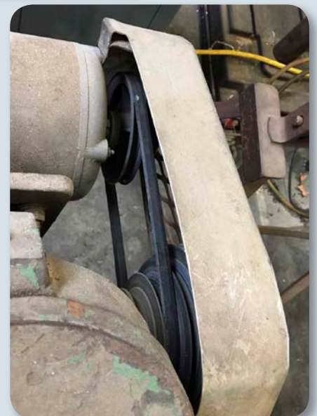
Photo 4: An older horizontal band saw that did not meet WHOI's requirement that safeguarding have an opening no larger than 6 mm (0.25 in.).
