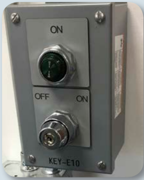
Photo 5: Key-operated selector switch that controls electric power to class 3 machinery.
